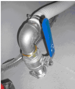
Discharge valve opened
