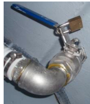
Discharge valve locked
